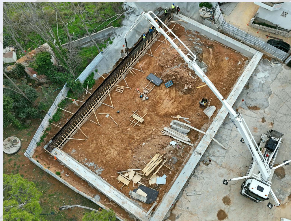
Concreting of the east side of the pile cap beam in DIKAIOSYNIS Shaft.
